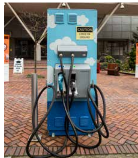
Electric vehicle charging station at Electric Avenue in downtown Portland
